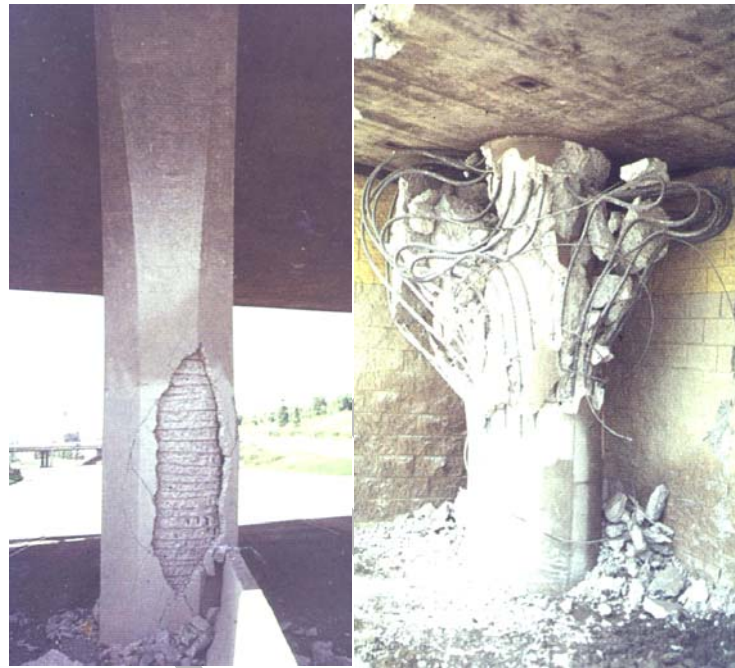
Fig. 1. Earthquake damage to a well-confined column and collapse of a poorly-confined column.
