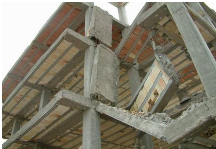
Figure 11. Poor performance of stairs in reinforced concrete structures
