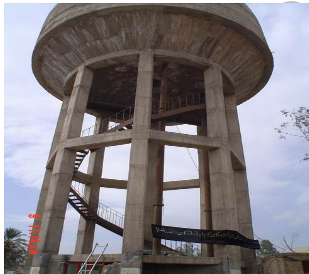
Figure 14. The elevated reinforced concrete water tank tower, where some cracks in the structural joints can be seen but the general performance is satisfactory.
