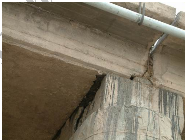
Figure 17. Separation of bridge Spans from the abutment
