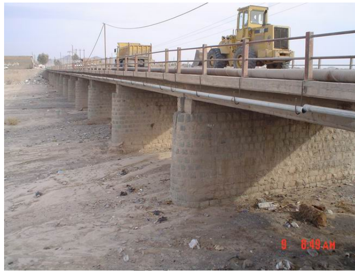
Figure 16. General view of the multi spans Reinforced Concrete Bridge after the earthquake which is in good condition and of course under service.
