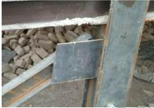
Figure 9. Incorrectly bracing with single I shaped brace only connected to the column
