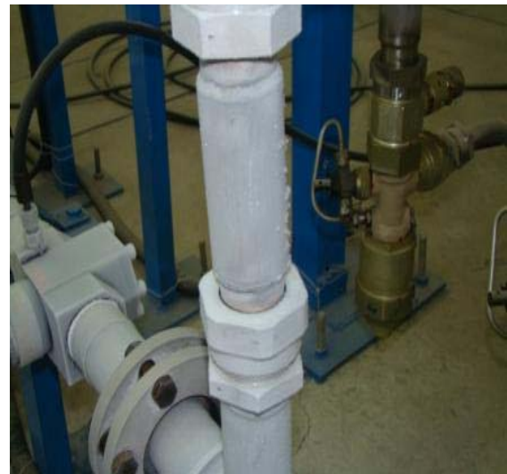
Fig. 2. Ice formed on the pipe after pressure regulation
